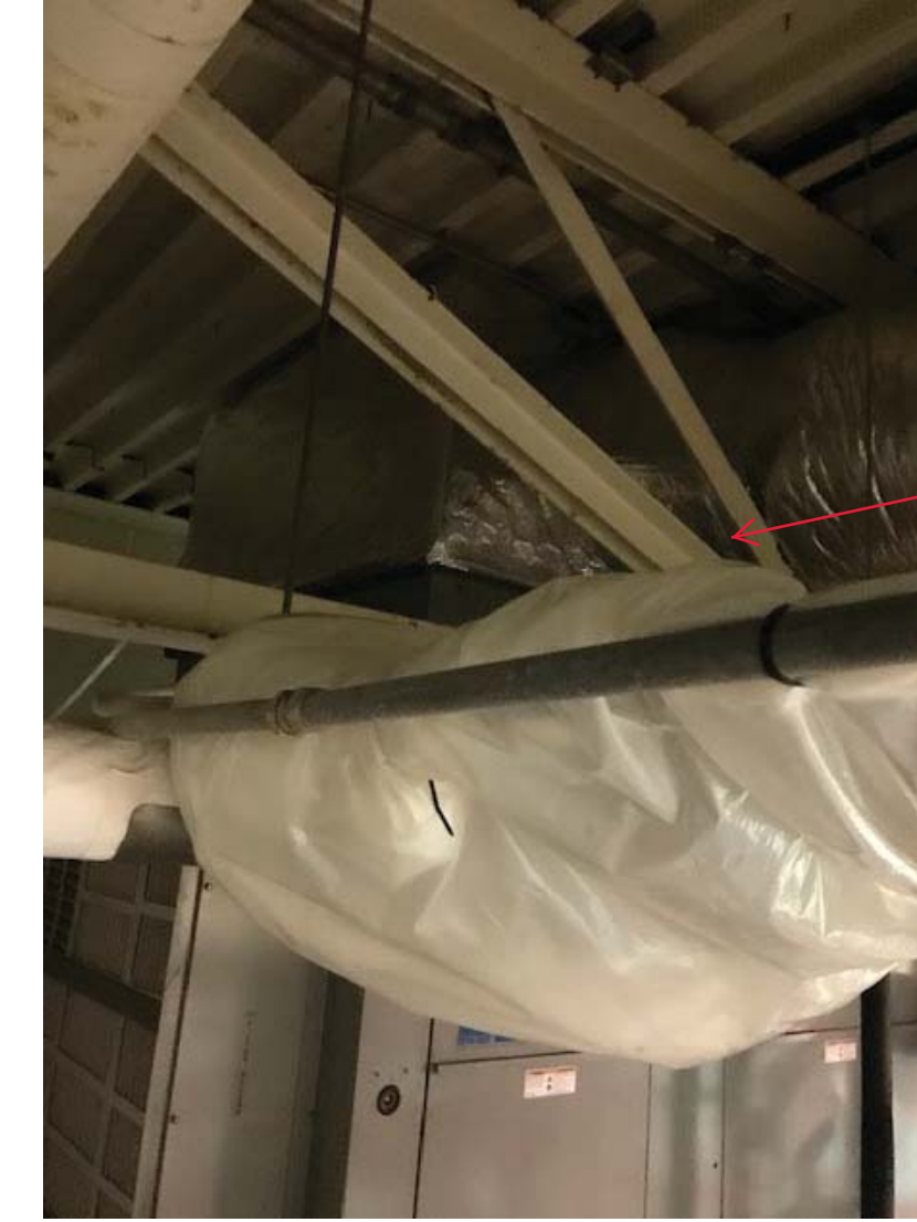
CONDENSATION PROBLEM UNDER OA DUCT
